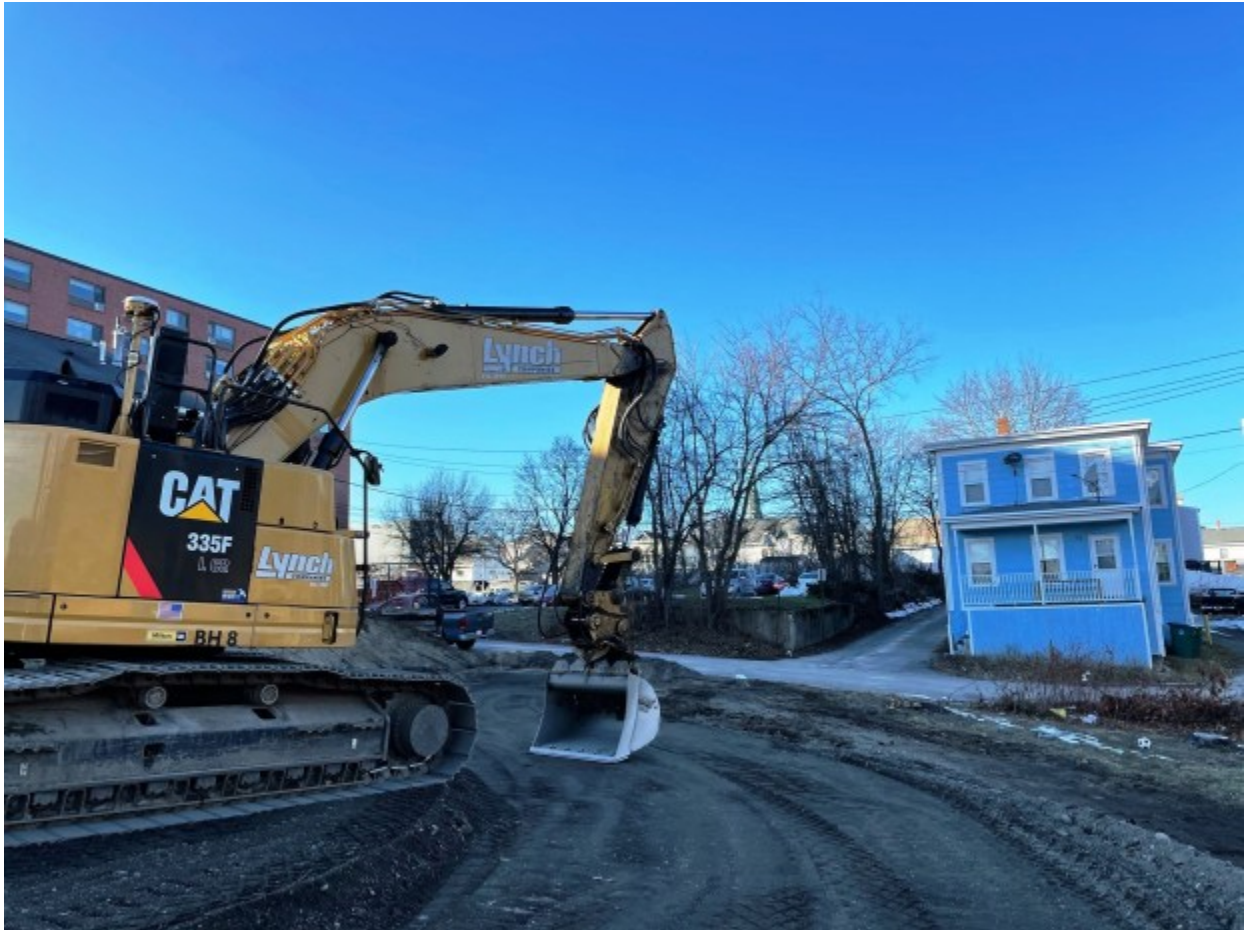
Making the grade where the rail trail will meet Fourth Street after passing below the Fifth Street Bridge in Fitchburg.
